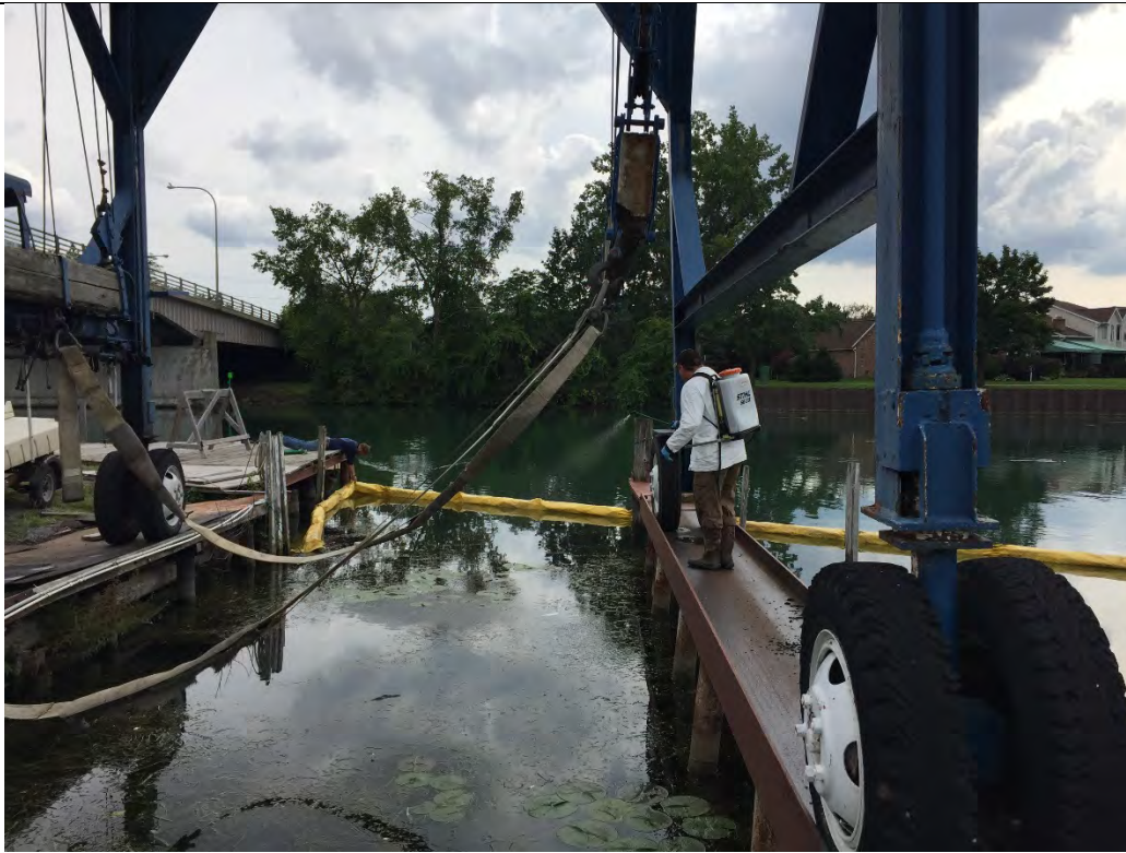
Date: 09/06/2017 Direction of View: West from North shore of creek Subject: SOLitude endothall sprayer application at Wardell Boat Yard Marina Description: Endothall was placed in the backpack tank and sprayed into the area around the marina by hand.
