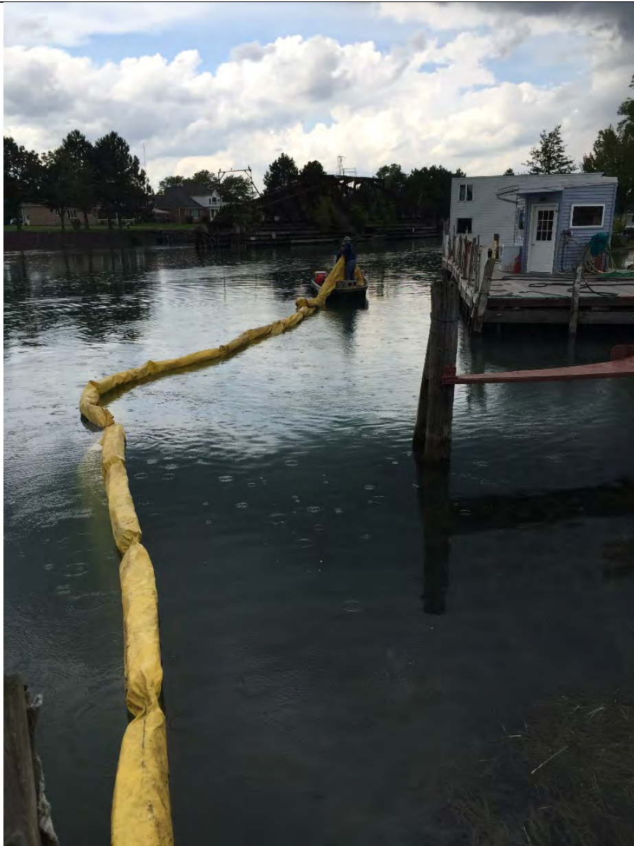
Date: 09/06/2017 Direction of View: West from North shore of creek Subject: Limnocorral at Wardell Boat Yard Marina Description: Installation of limnocorral at Wardell Boat Yard marina for isolated spraying of endothall from shore by backpack and from boat.
